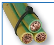
Nylon Cable Tie Tensioned/Cut/No sharp edges
