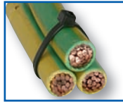
Nylon Cable Tie Tensioned/Cut/No sharp edges
